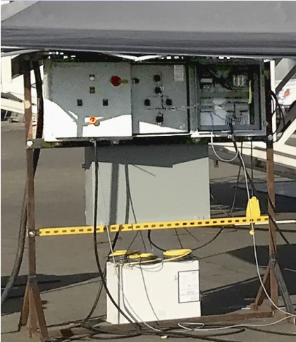
Custom-built Duff-Norton Automated Actuator System (AAS) in staging area.
